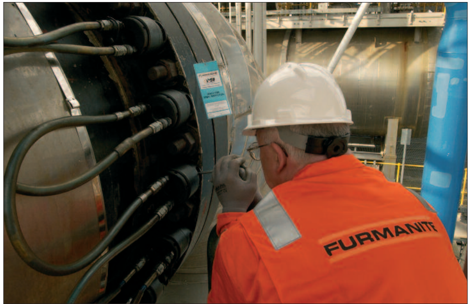
Ensuring joint integrity requires a certain level of engineering and management - simply installing a gasket and tightening the bolts will not guarantee a reliable, leak-free joint.
