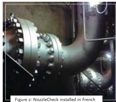
Figure 2: NozzleCheck installed in French nuclear power plant
